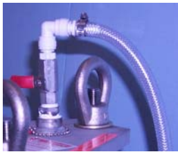
Air purge valve and drain tubing
