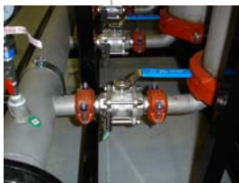
Stainless Steel Manifold with Stainless Steel Valve
