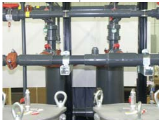
PVC Paint Manifold
