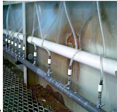
• Typical Industrial ED System Electrolyte Manifolds
