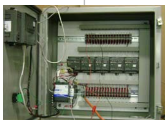
Interior view of panel
